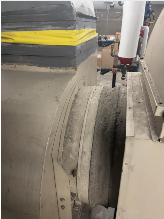
Figure 11: General view of horizontal surfaces with accumulated dust/debris present within Fan Room around ductwork (typical).
