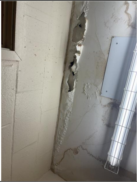
Figure 9: General view of peeling paint and efflorescence on plaster ceiling within assessed areas.
