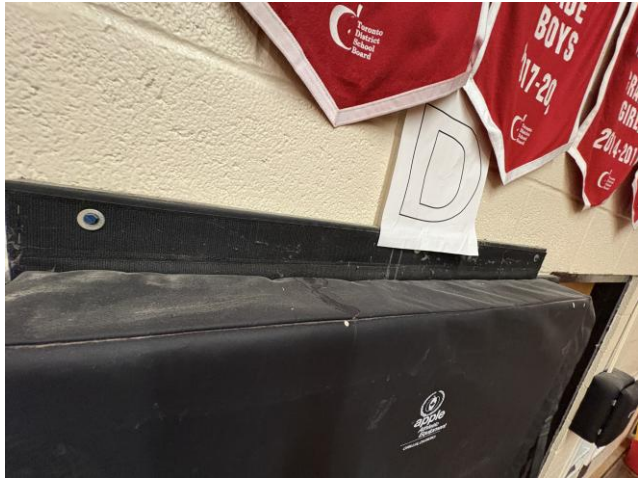
Figure 3: General view of horizontal surfaces with settled dust/debris in the Gym (typical).
