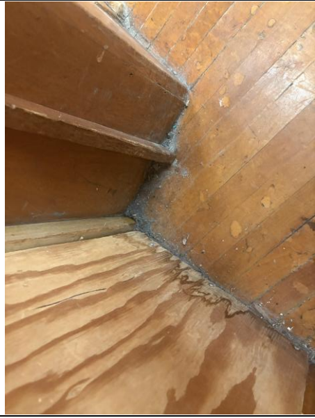
Figure 10: General view of horizontal surfaces with accumulated dust/debris present within Gym (typical).
