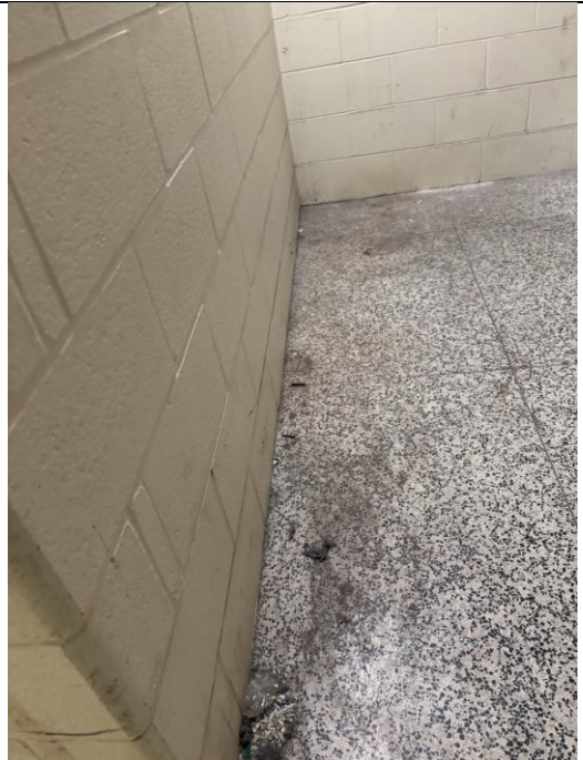
Figure 12: General view of horizontal surfaces with accumulated dust/debris present within Fan Room.
