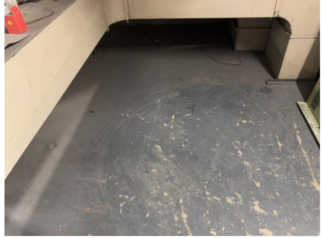
Figure 6: General view of horizontal surfaces with accumulated dust/debris present within Fan Room around ductwork (typical).
