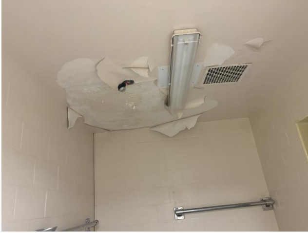
Figure 5: General view plaster ceiling within Boy's Changeroom.
