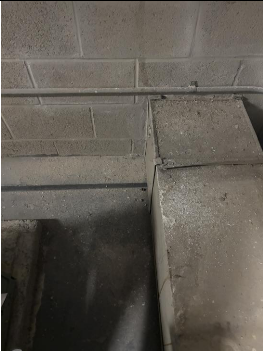
Figure 7: General view of horizontal surfaces with accumulated dust/debris present within Fan Room around ductwork (typical).
