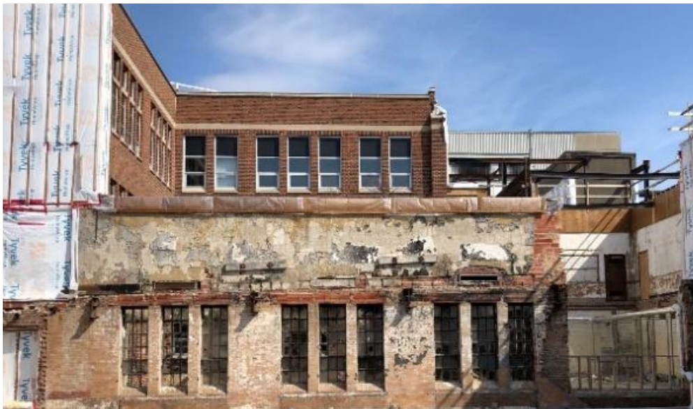
Post-fire view of dismantled east auditorium wall.
